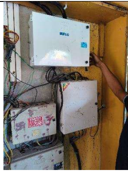
Photo: Incomer from C.O.-2 input side (direct Grid connection)
