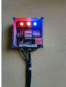
Photo: Output switch of the Solar Inverter
