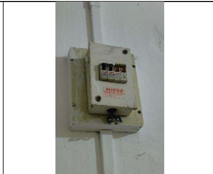
Photo: DB at Electronics Lab Classroom
