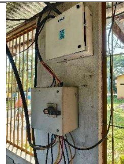
Photo: Grid / DG-2 Changeover (C.O.-2)
