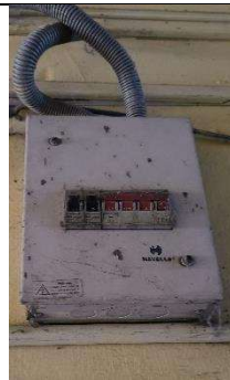
Photo: IQAC AC DB (Admin Bldg. GF)
