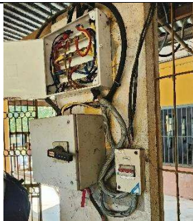
Photo: Grid / DG-1 Changeover (C.O.-1)
