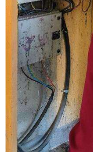
Photo: Incomer from the Solar Inverter
